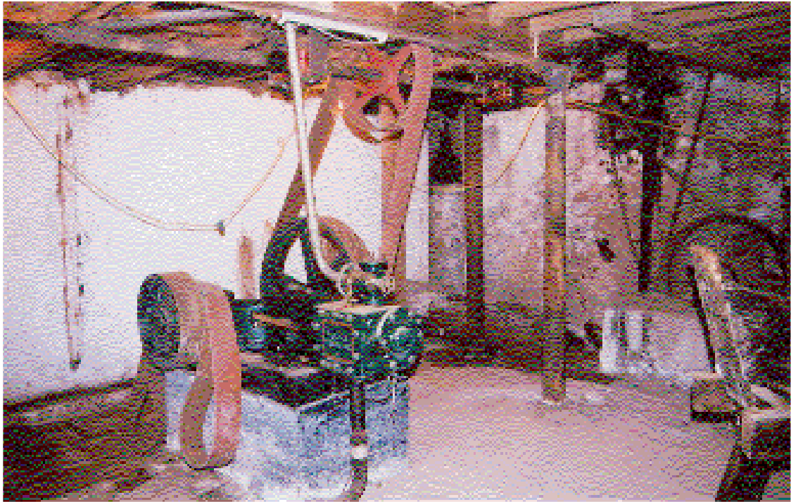
Plate 17. Tangye Steam engine and water wheel enclosed behind the wall, Building 4, Basement, Looking SE.
